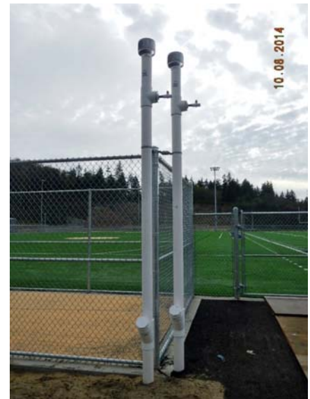
Gas monitoring vent and sample port
